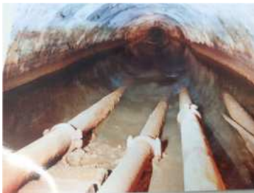
Underwater pipes leading into the water lodge
